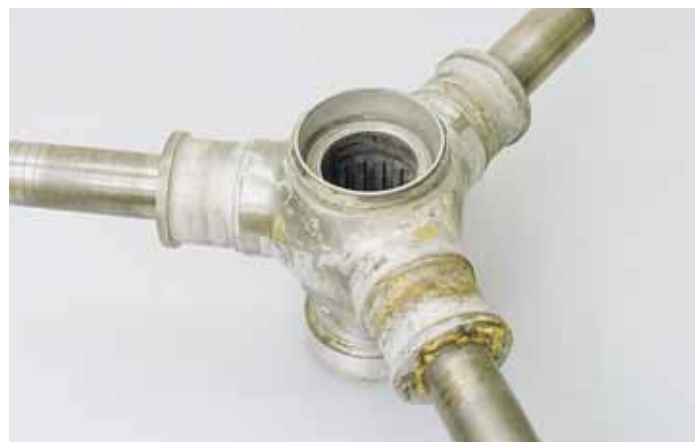
Corroded steel hub
